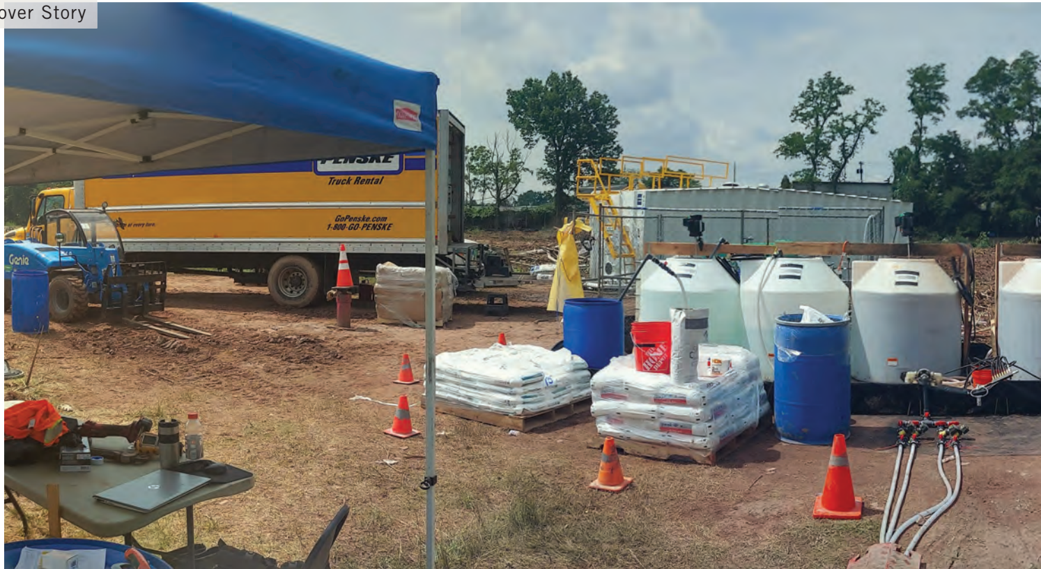
Injection pumps and mixing tanks are used to conduct in-situ chemical oxidation of contaminants at Bridge Industrial's project in Belleville, New Jersey. The site is within six miles of the Lincoln Tunnel, a major artery into New York City.
