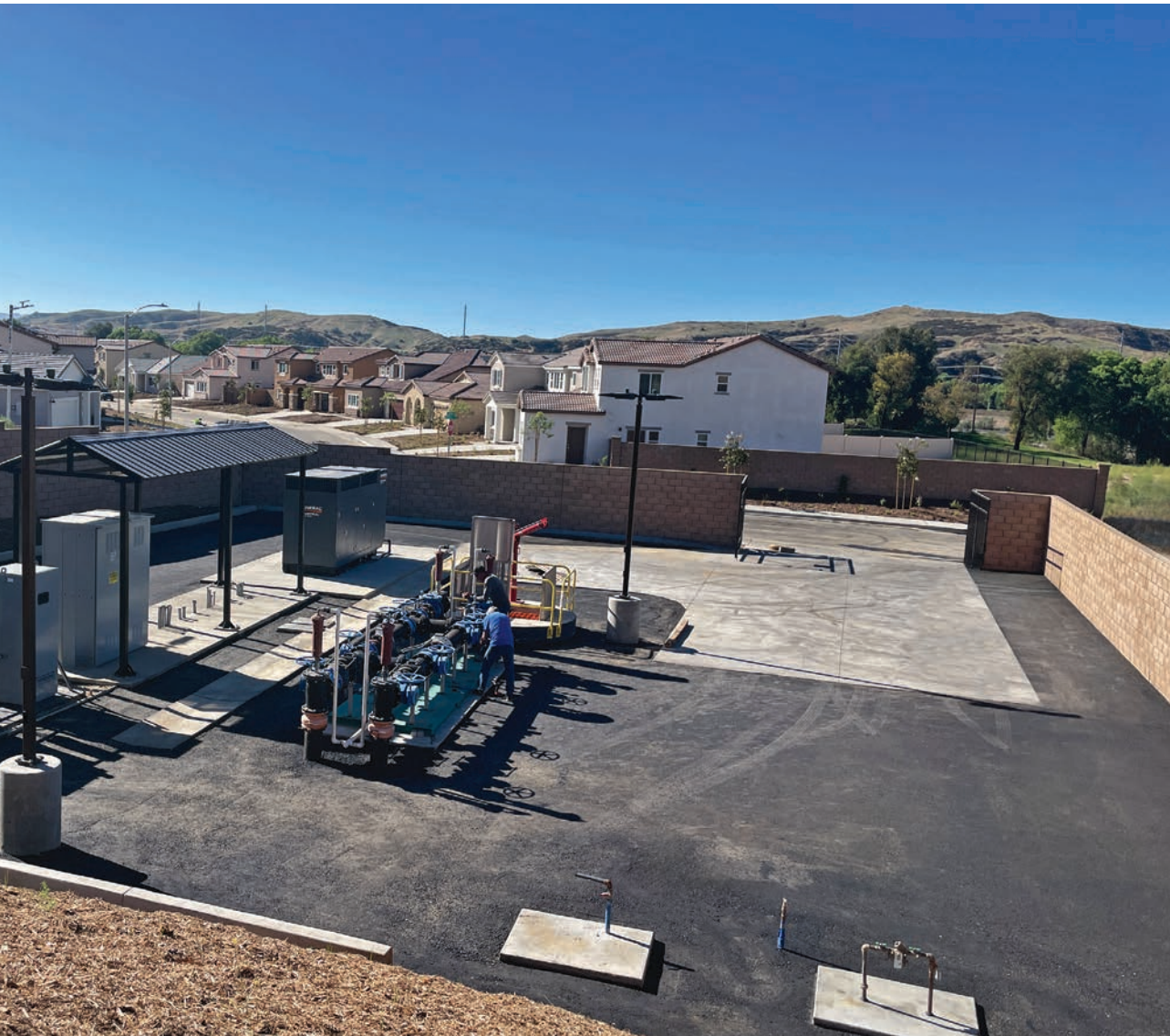
A phased residential wastewater lift station can accommodate both current and future flows as the residential area expands.
