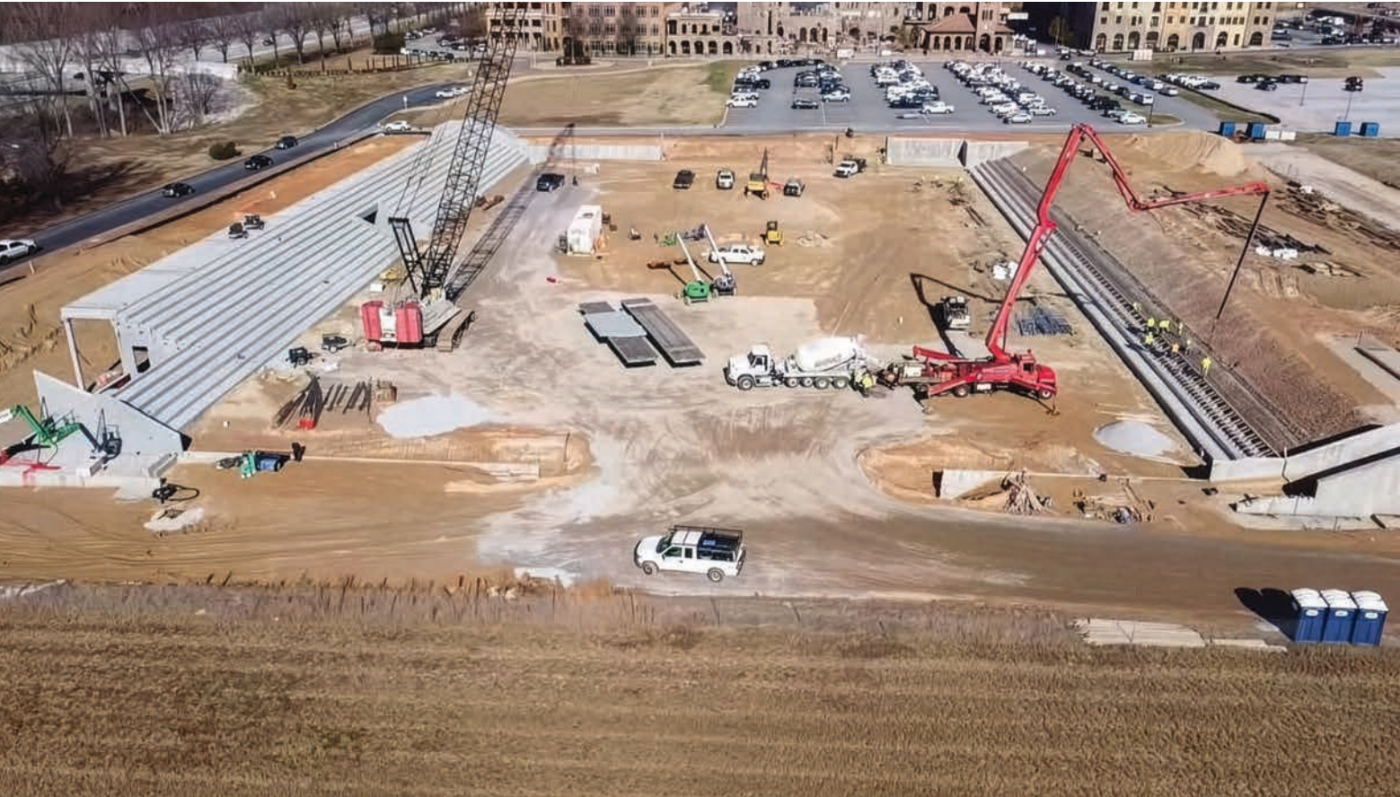
The in-progress GE Vernova Park at BridgeWay Station, a mixed-use development in the growing upstate region of South Carolina, will serve as the future home of the Greenville Triumph and Greenville Liberty soccer teams.
