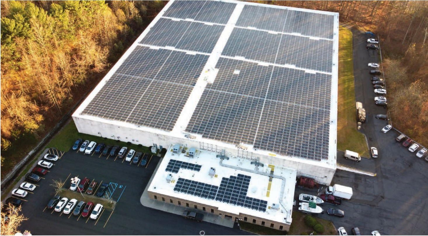
The Mines Press plant in Cortlandt Manor, New York, features a battery energy storage system.
