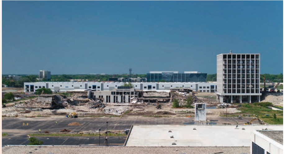
Concrete and asphalt gathered during demolition were ground up and used as fill on The Logistics Campus.
