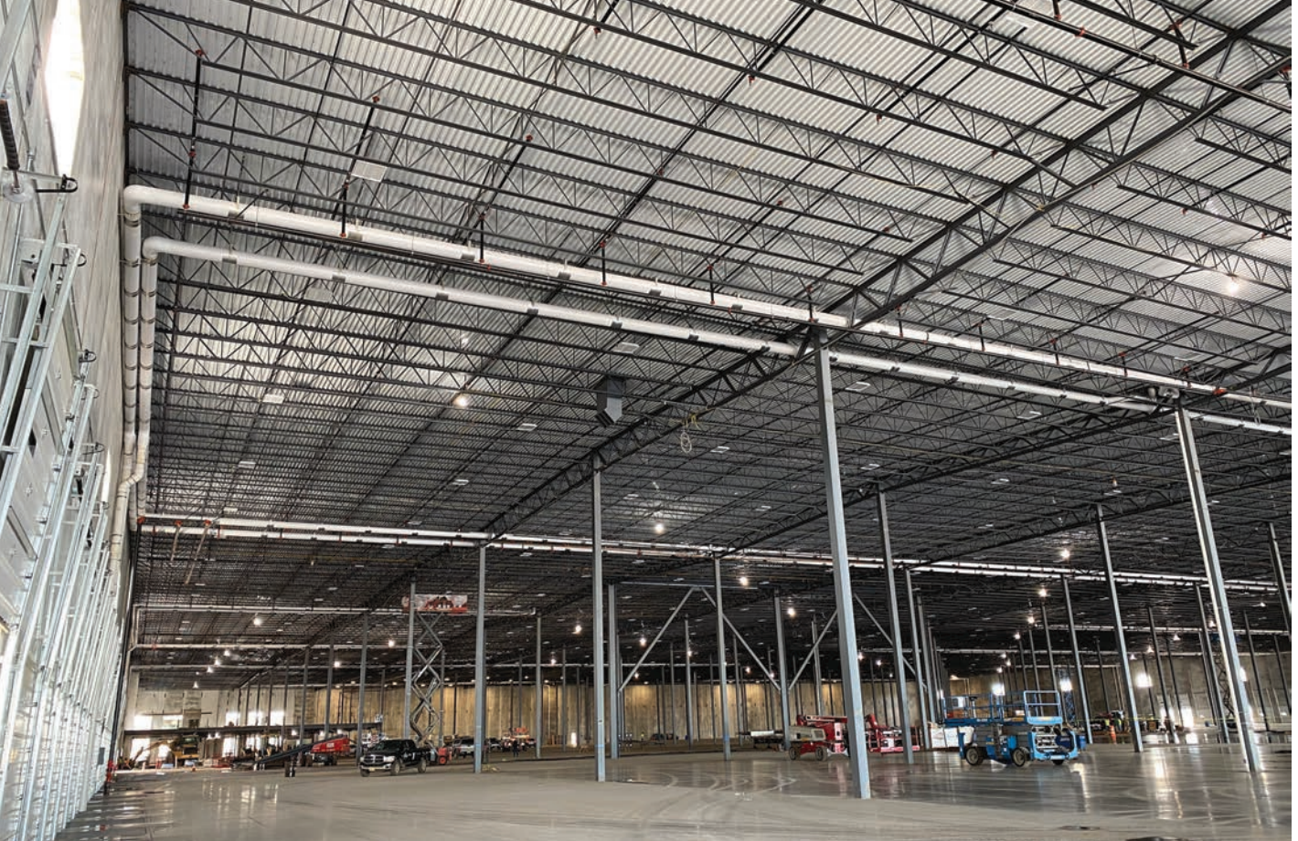
A siphonic roof drain system inside an industrial building. These systems allow for greater flexibility when it comes to the placement of pipes.
