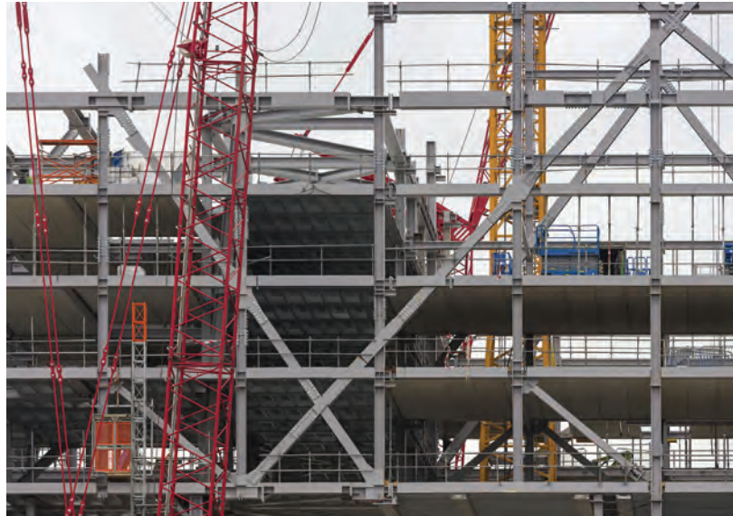
Construction loan monitoring (CLM) aims to root out problems on a project at the early stages before they can get bigger and costlier.
