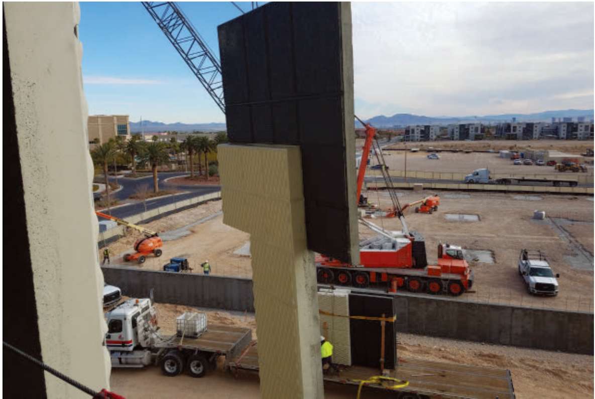
A section of the precast concrete panels for Two Summerlin is moved into place at the job site.
