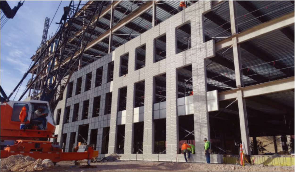
The precast concrete panels at Two Summerlin are attached to a steel frame structure. Inserts in the panels and rods in the inserts tie the concrete together.
