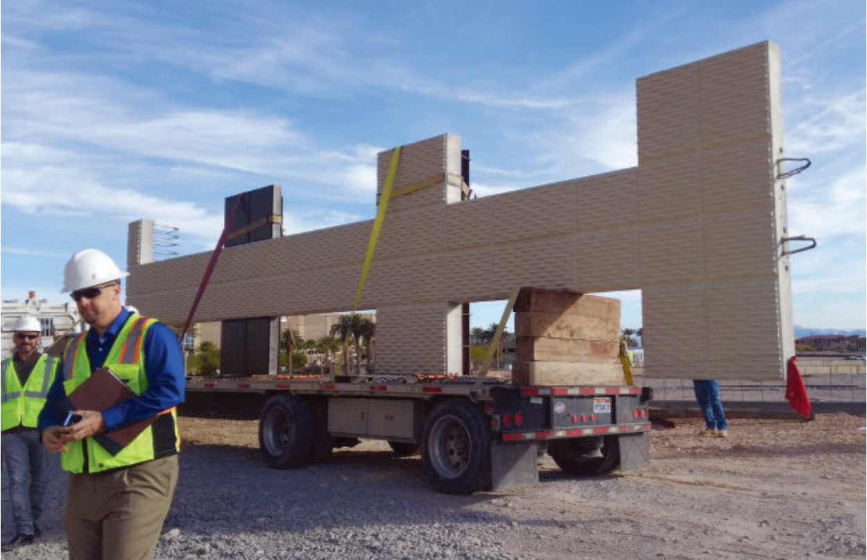
Precast concrete panels were used for the exterior of Two Summerlin. According to The Howard Hughes Company, it marked the first time this application has been used in Nevada.
