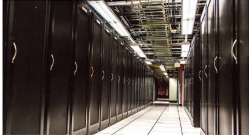
West 7 Center's Tier III data center facility occupies three underground levels.
