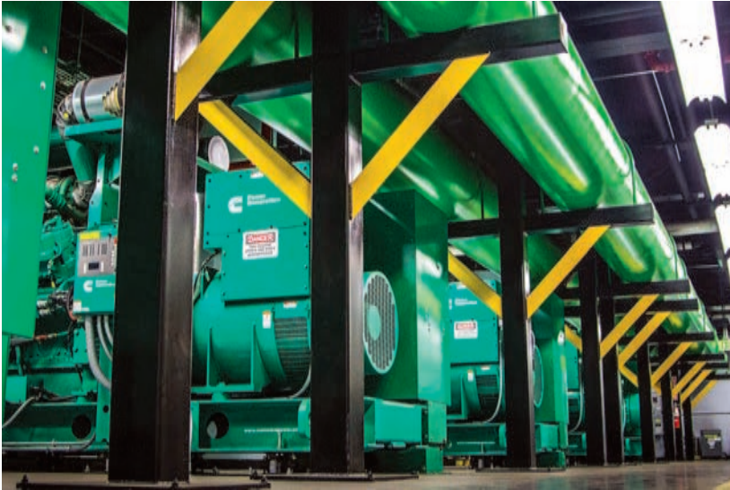
The building's emergency generator plants feature five 2,250 kW, four 1,100-kW and one 1,250 diesel generators, resulting in 16.9 mW of total capacity. It is supported by three 30,000-gallon underground fuel storage tanks designed to support the building's critical infrastructure at full load for approximately 120 hours.
