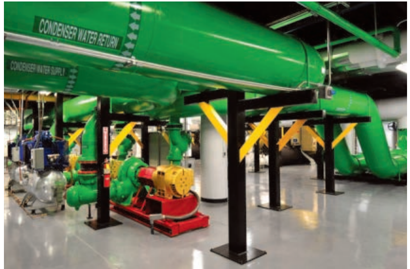
West 7 Center's chiller plants feature four 1,250-ton, three 1,000-ton and two 500-ton centrifugal chillers, resulting in 9,000 tons of total cooling capacity. They're served by nine cooling towers.
