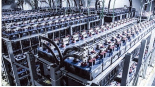
The building's battery farm provides a 3,750 kVA uninterruptible power supply (UPS) for critical functions.
